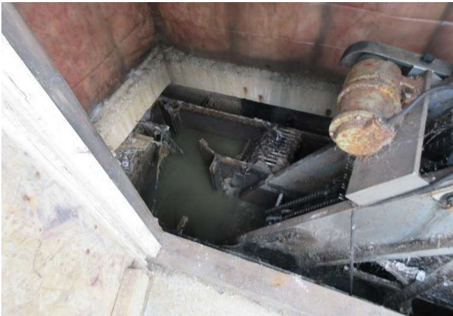
Interior debris screen
