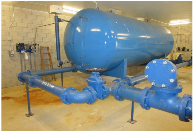
Tank and piping
