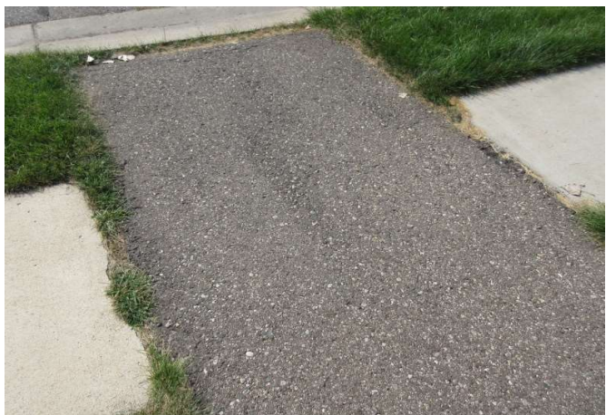
Settled walk at street
