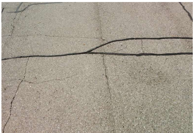
Cracks and crack repairs
