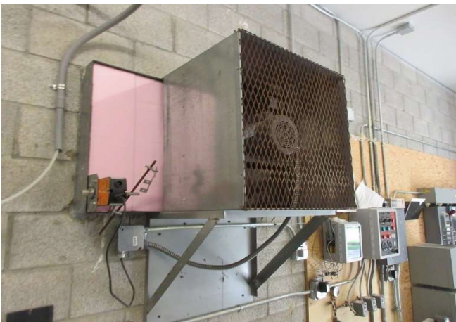
View of fan
