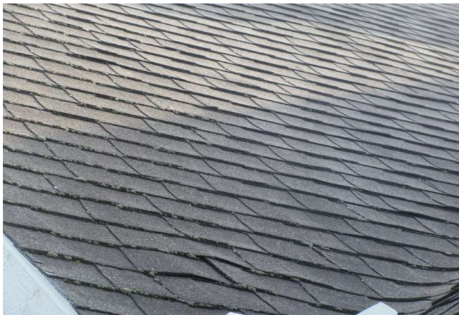
View of minor shingle lift and organic growth
