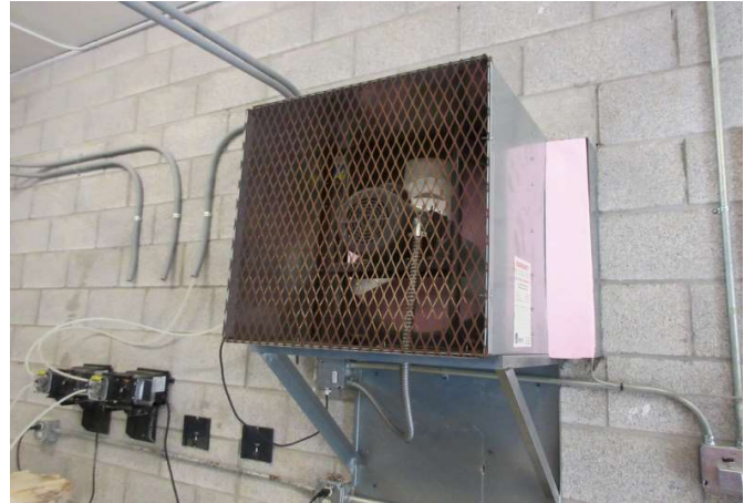
Exhaust fan at pumphouse
