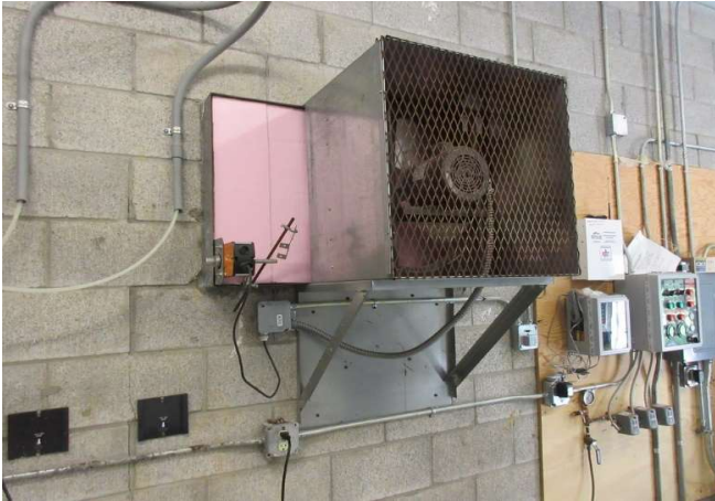
Fan in pumphouse
