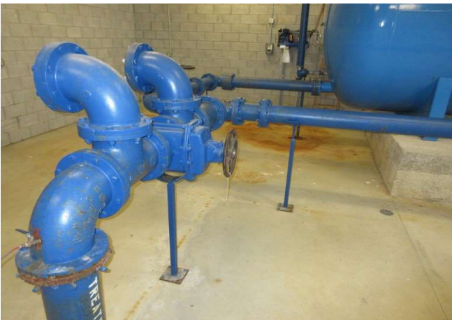
Piping at tank
