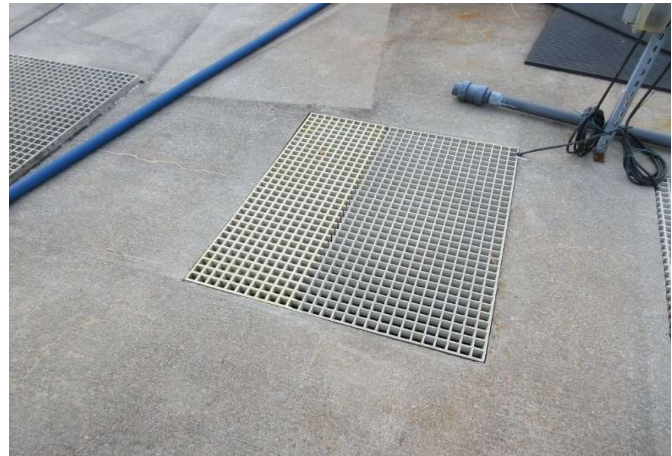
View of access panel
