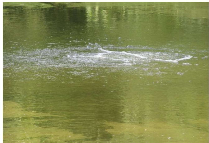
Bubbler aerator in small pond
