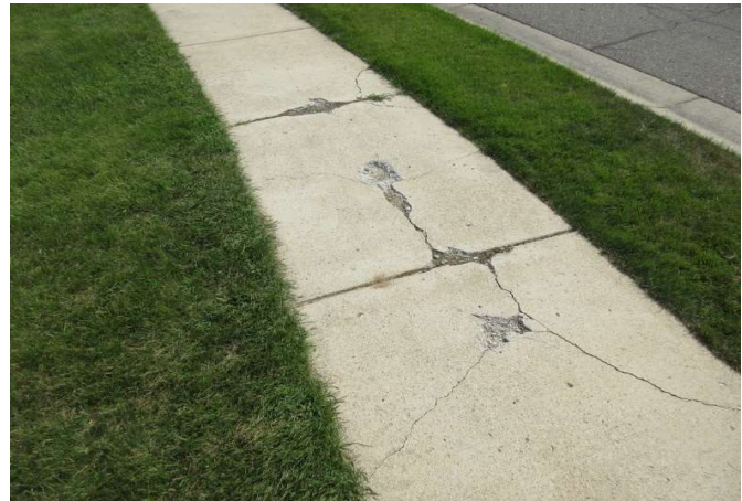
Cracks in walk
