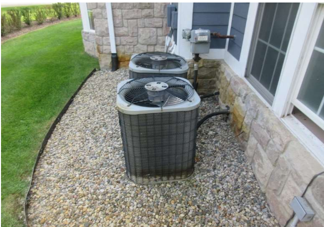
View of condensing unit
