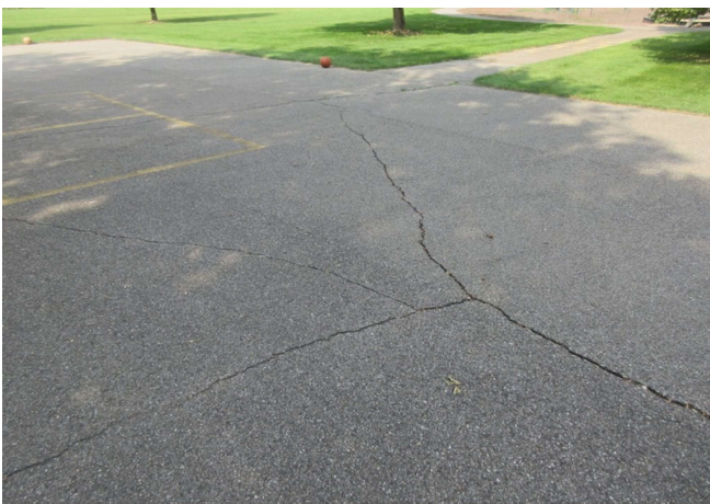
Cracked asphalt basketball court
