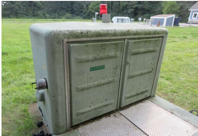
Lift station cover
