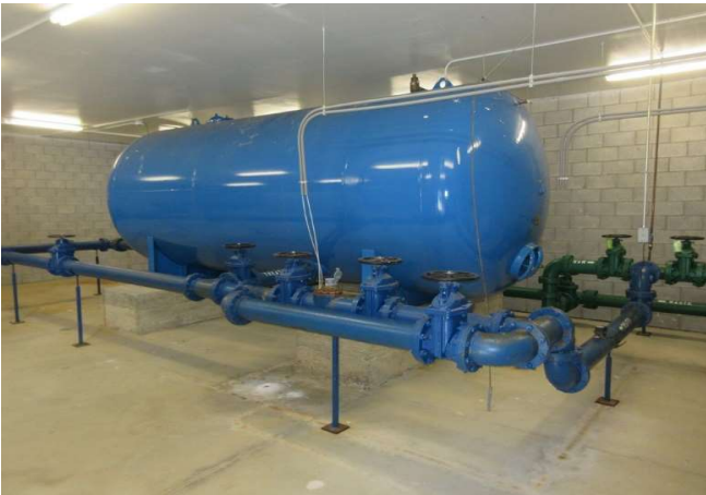
View of tank
