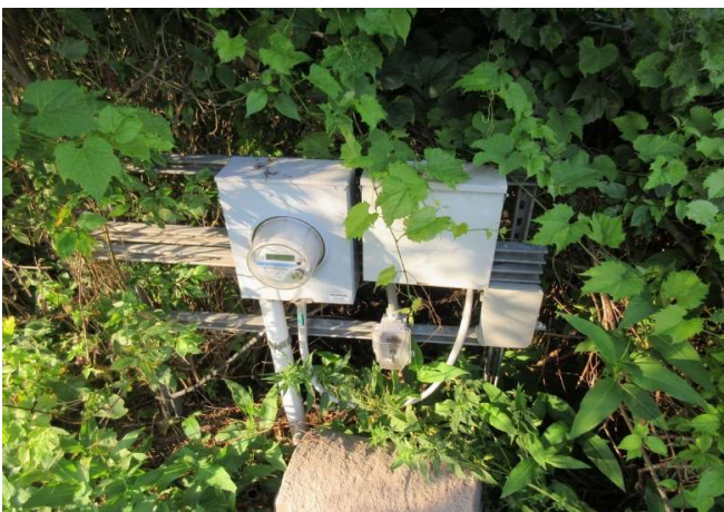
Aerator control panel
