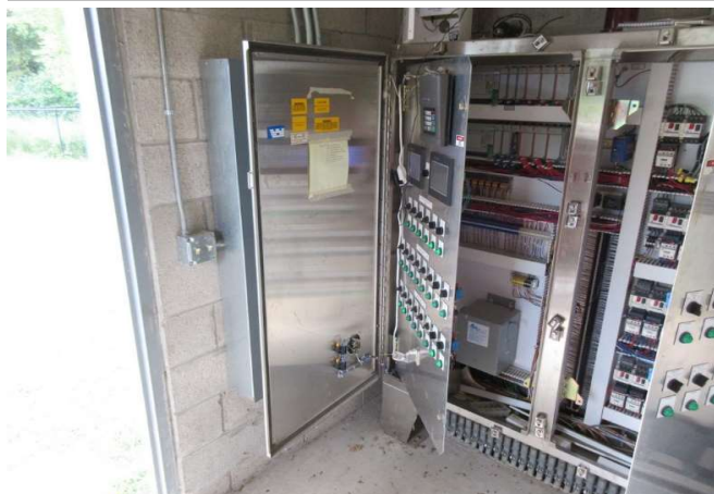
View of alarm panel
