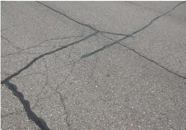
Crackle and repairs
