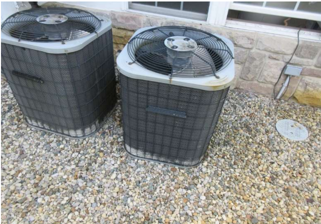
Condensing units at clubhouse
