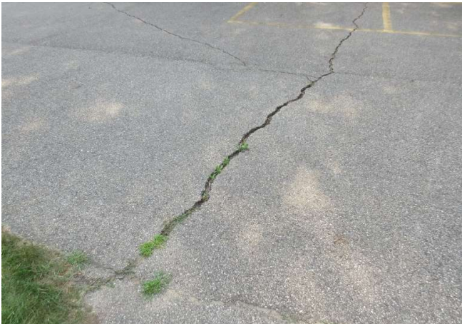
Crack in court
