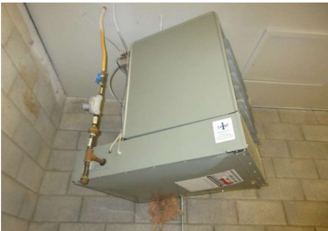
View of gas line
