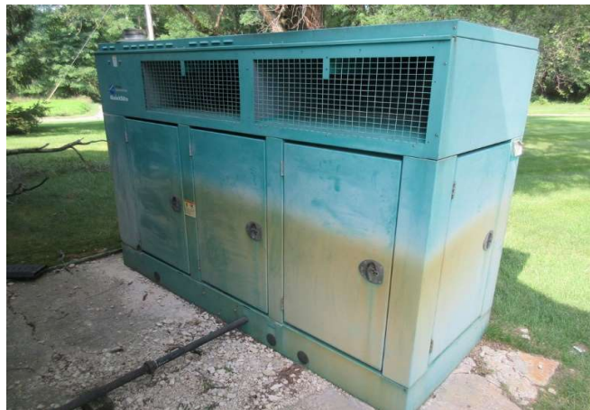
Generator at wellhouse
