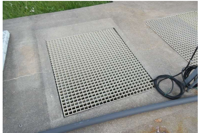
Vented treatment system hatch
