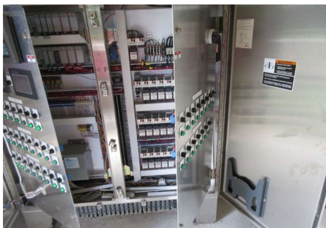
Panel was open during inspection
