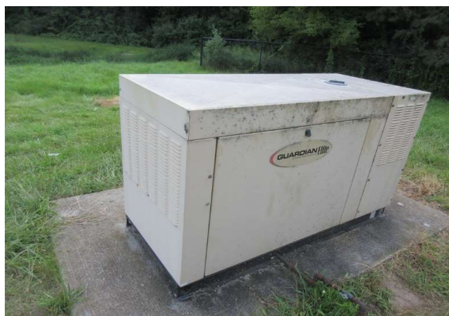
Generator near pumphouse
