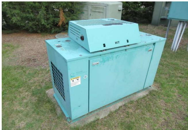
Generator at lift station
