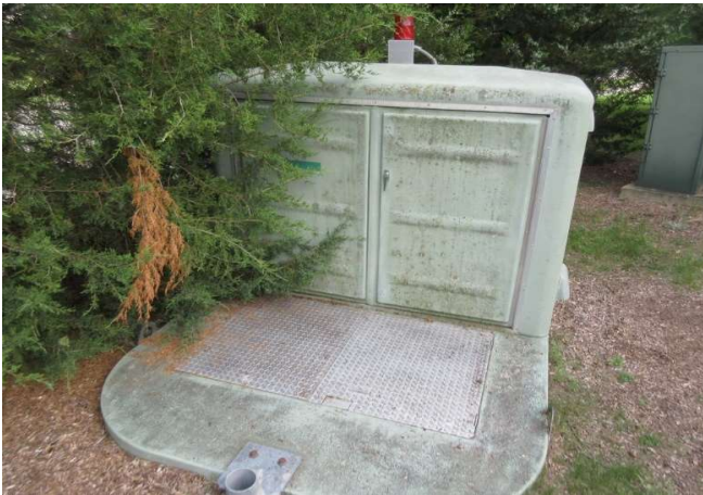
Typical lift station
