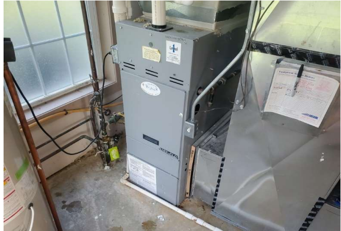
AHU in mechanical room
