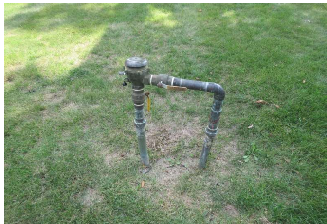
Irrigation valve near wellhouse
