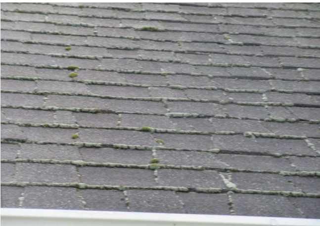
Organic growth on roof
