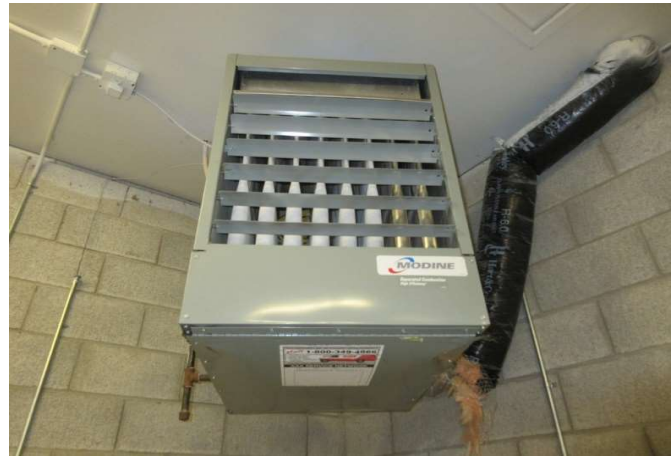
Ceiling mounted heater
