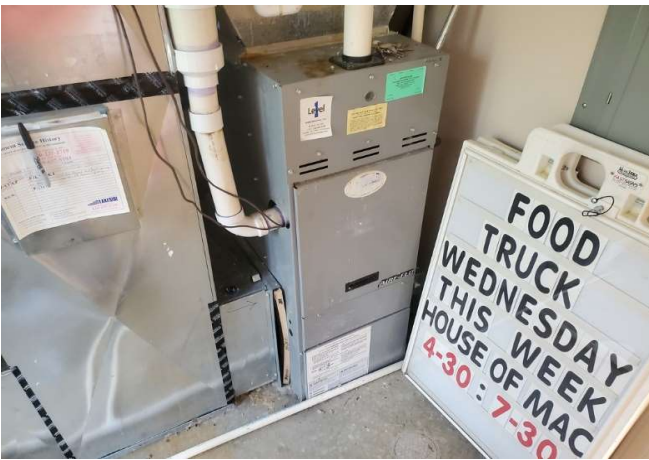
View of furnace
