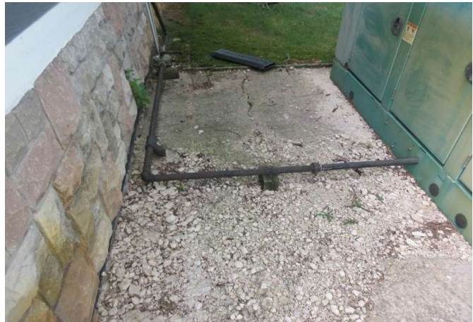
Pad deterioration at generator
