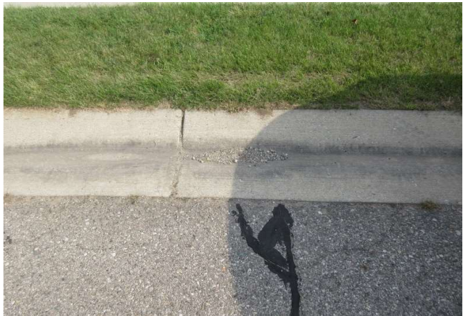
Curb with debris
