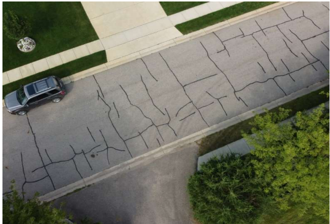
Aerial view showing cracking
