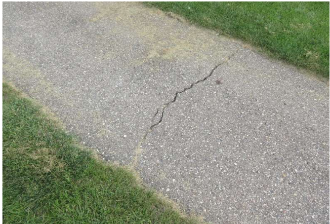
Crack in walk
